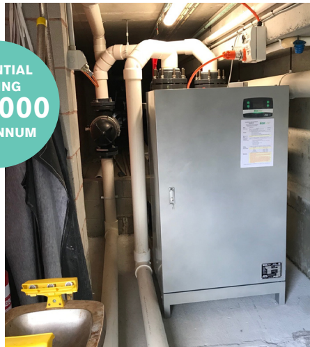
Southern Cross University backwash reduction project - freshwater chlorinator
