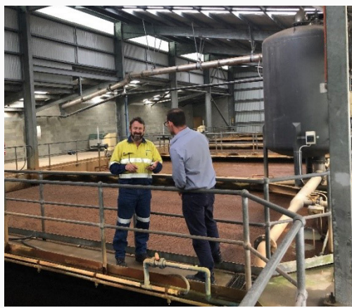
All assets in the Nightcap Water Treatment Plant are in good condition.
