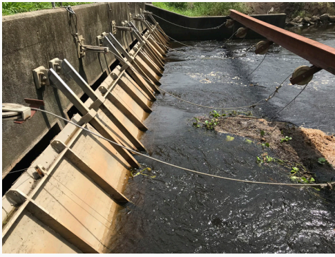
Blackwater discharging from the drainage system into the Richmond River estuary following La Nina flooding event.
