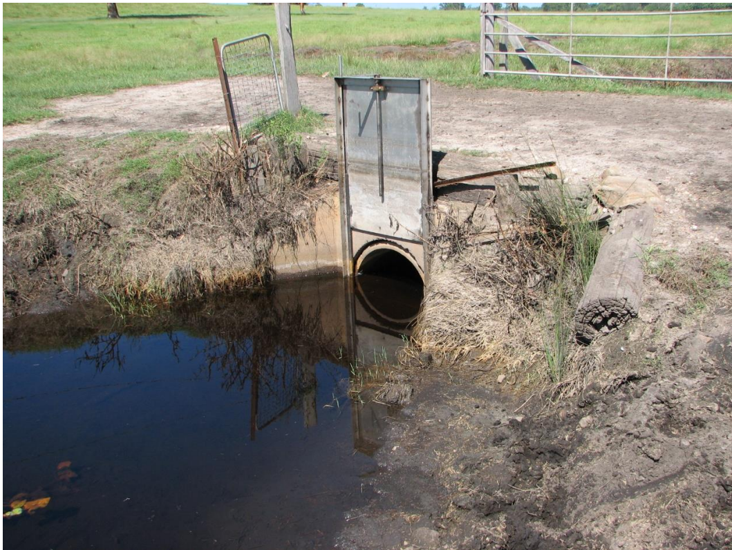
4: Slide dropboard that was fitted to the private piped crossing to hold drain water levels up above stream.
