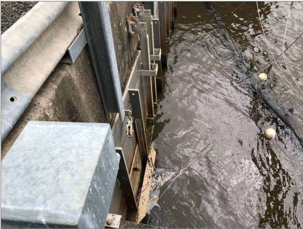
Figure 3: Sluice window installed on the floodgates at North Woodburn-Kilgin drain.
