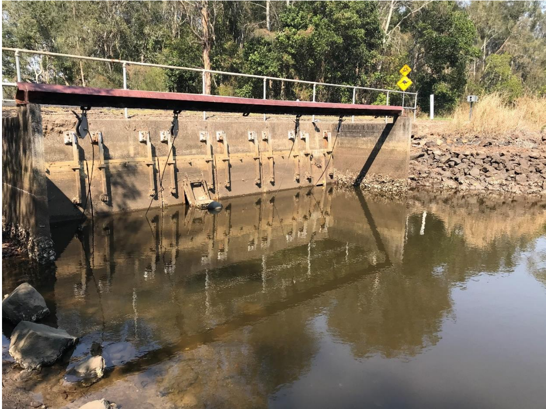
3: KHDS floodgates, showing the automatic tidal float mechanism and new sluice window on the far right floodgate.
