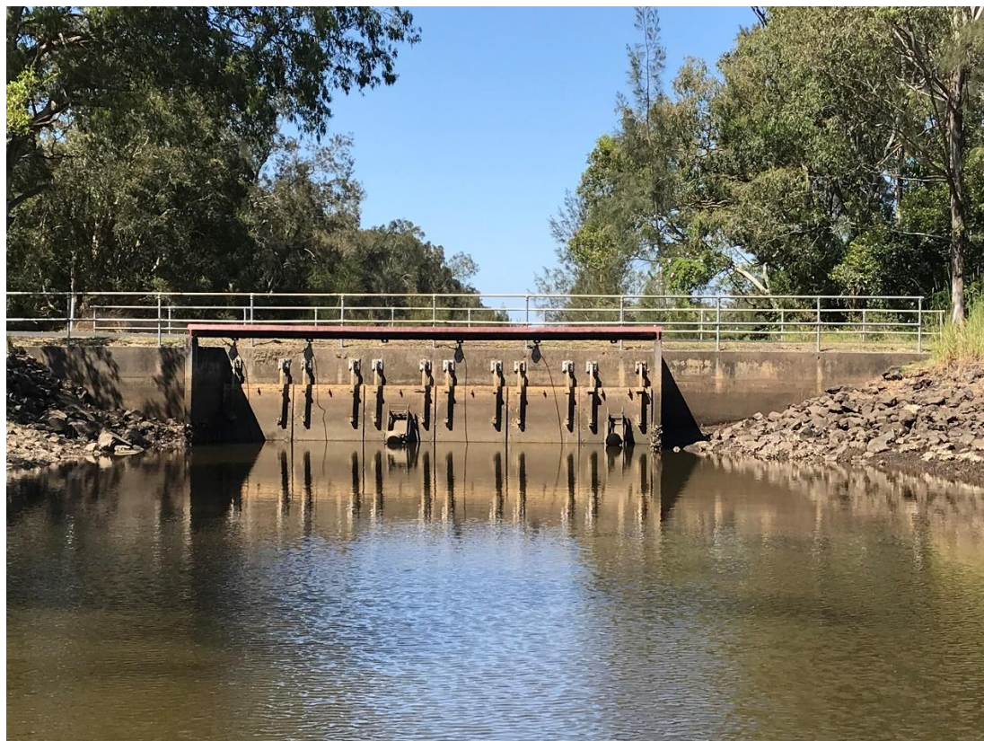
2: KHDS floodgates, showing two previously installed automatic tidal float mechanisms.
