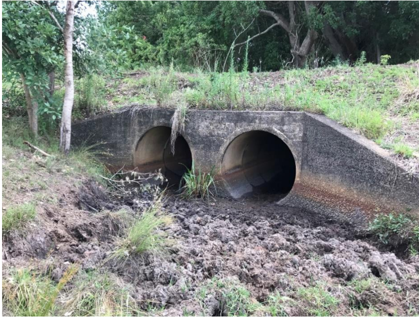
12: Historic culvert and levee on south-west upper arm of creek, looking downstream.
