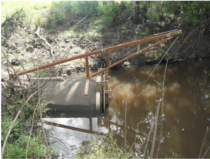
2: Bora Creek floodgate and lifting gear in operational position.
