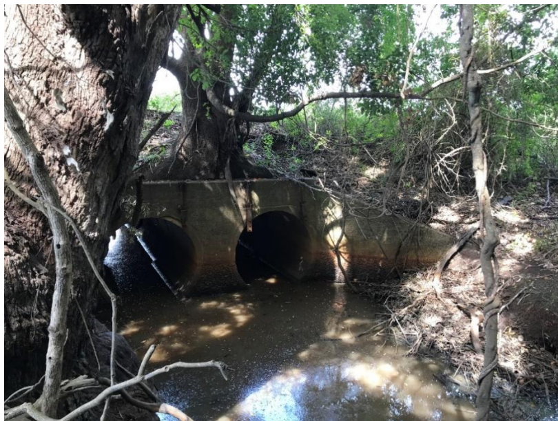
11: Historic culvert and levee on south-west upper arm of creek, looking upstream.
