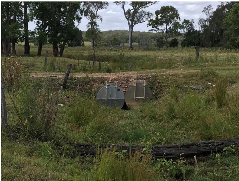
13: Council managed floodgates (asset number 1975) on upper south-west arm of Bora Creek.
