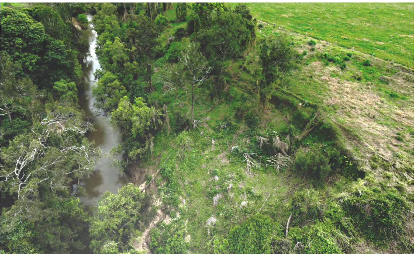
Figure 124. Example of large rotational mass failure that has self-stabilised with time post initiation.
