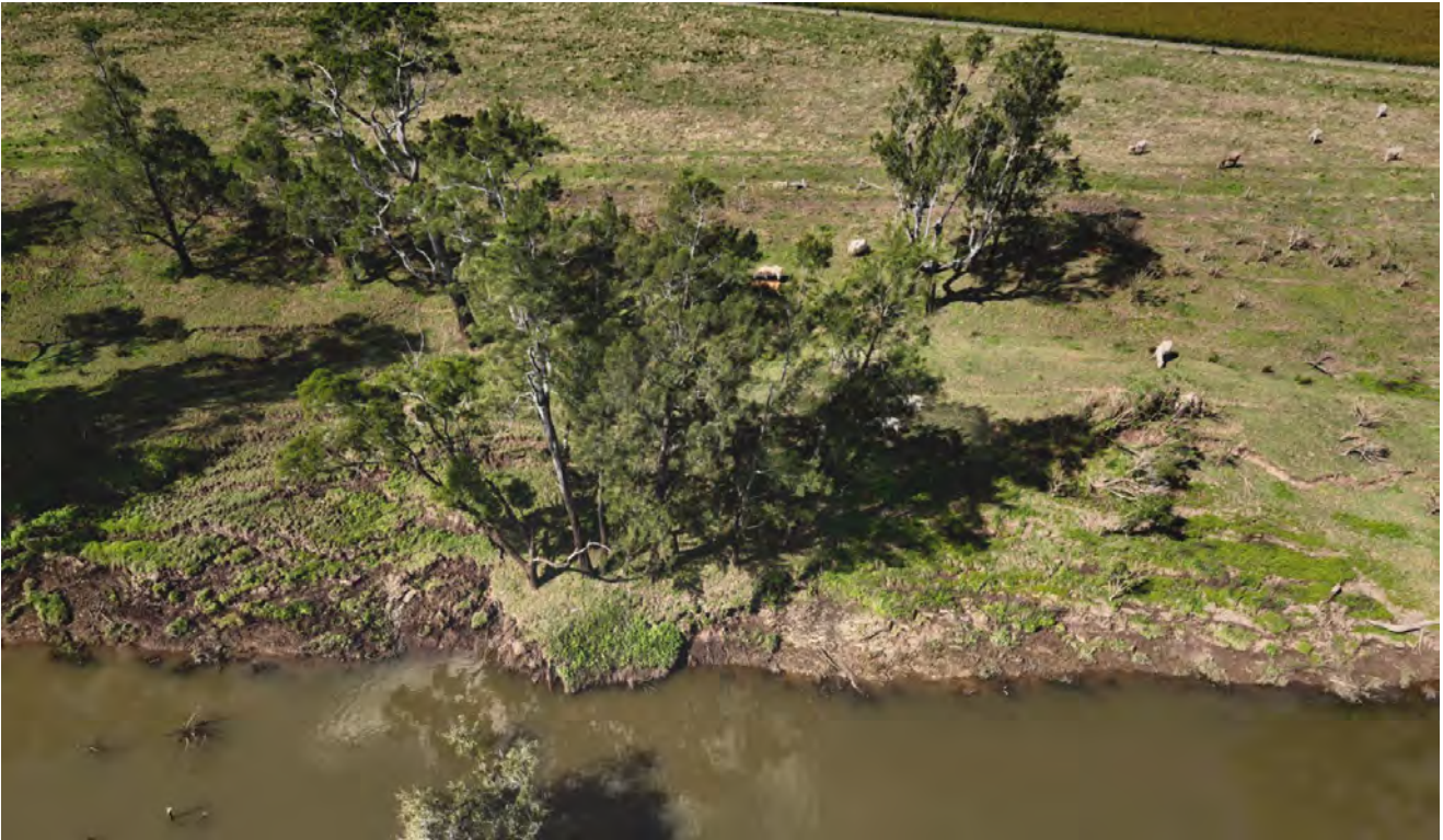
Figure 125. Toe scour along a devegetated section of river, in which the only section of bank toe not scoured is the section associated with the root mat of the Casuarina cunninghamiana. A river reach like this would benefit significantly from stock exclusion.
